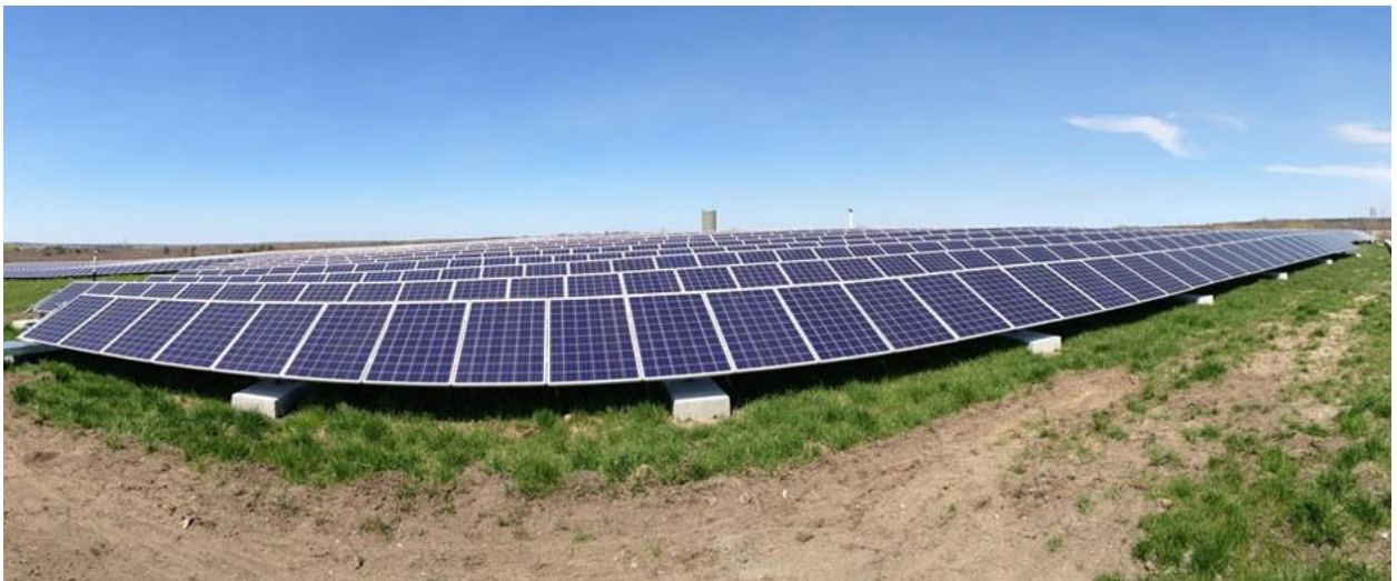
TYPICAL LANDFILL BALLASTED SOLAR ARRAY
